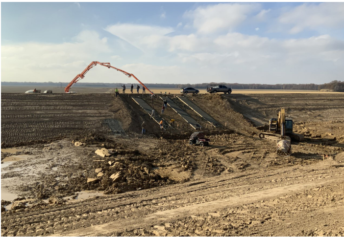
Preparations for the installation of water control gates at a landowner offtake.
